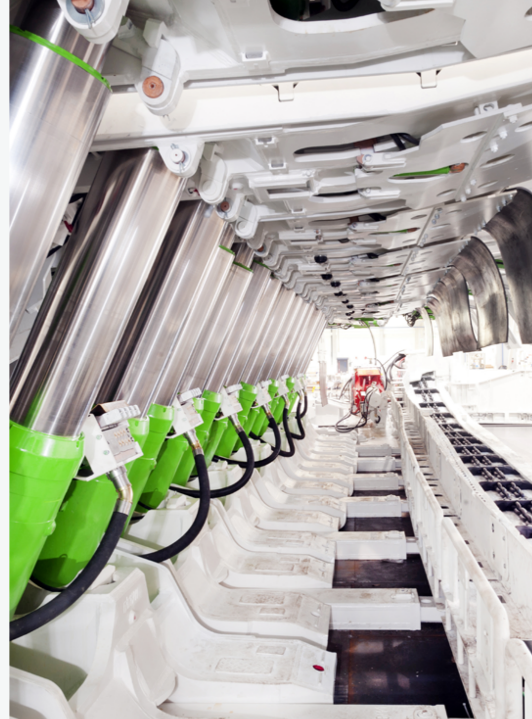
➤ Powered roof support system
